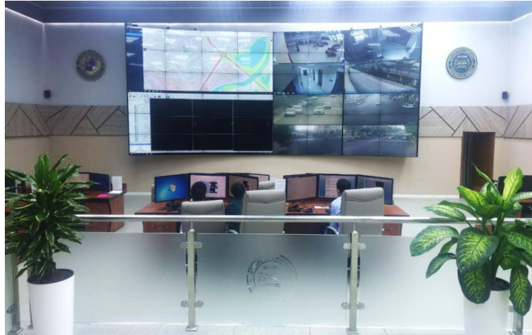
Figure 4. Central control panel in the city of Jizzakh (U. Torakulov street 24, Jizzakh city).
