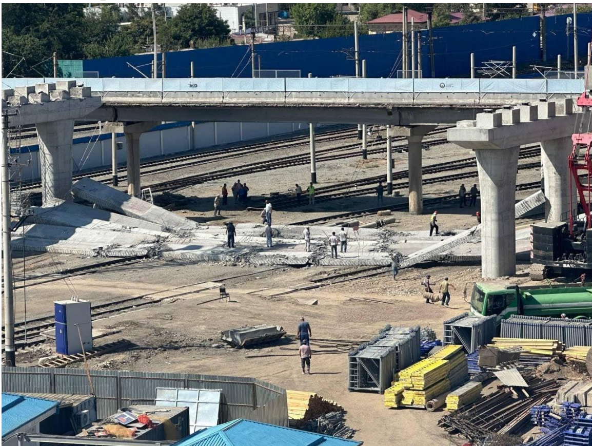
Picture 2. Five beams of an overpass under construction near the airport in Tashkent collapsed.
