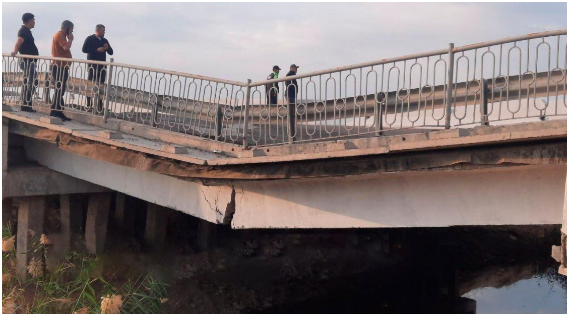
Picture 1. In the Akaltin district of the Syrdarya region, a bridge broke and the road collapsed.
